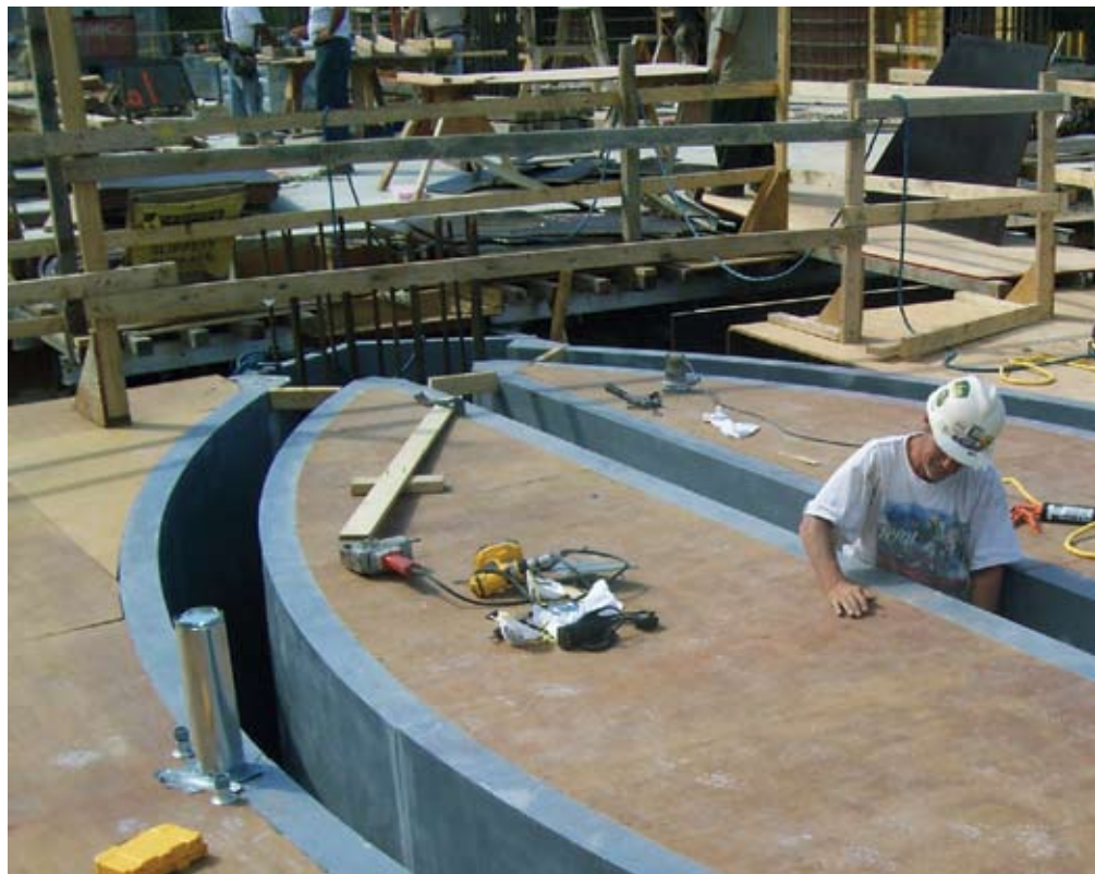
Fig. 3: Formwork for the entryway was reassembled on site and integrated with the soffit formwork for the floor slab for the level above
