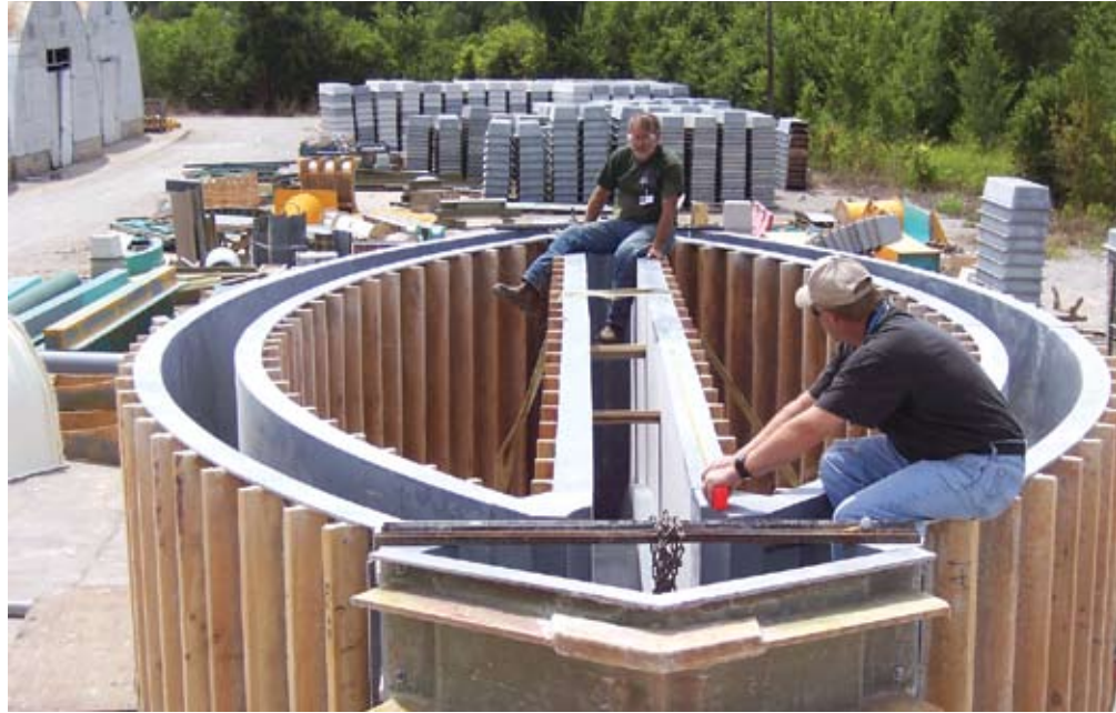
Fig. 2: Prior to shipping to the job site, workers assembled formwork for the entryway to check fit and dimensions. Note dimension lumber and plywood studs bonded to the fiberglass sheathing
