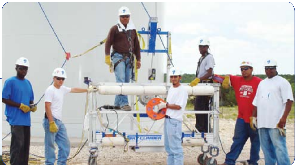
The Wind Energy Services Team employs an interesting wind cage to repair turbine blades without expensive cranes or removing blades from the rotors. WES team members shown making repairs at the Sweetwater, TX Phase III wind farm.
